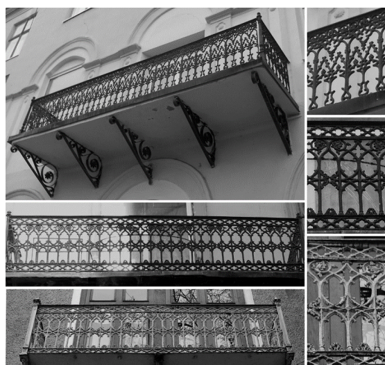
Fig. 4. Cast balcony fencing on the buildings situated at: 29, Halytska Str. (dated 1835); 2, Bachynsky Str. (dated 1874–1880); 4, Shevchenko Str. (dated 1880th)
