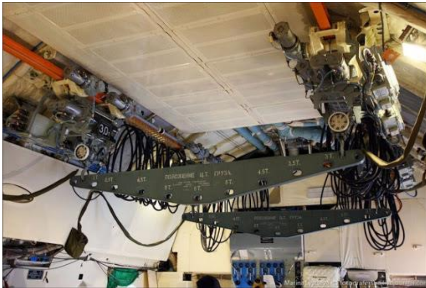
Fig.2.1(a). – Telfers in Il-76 cargo compartment
