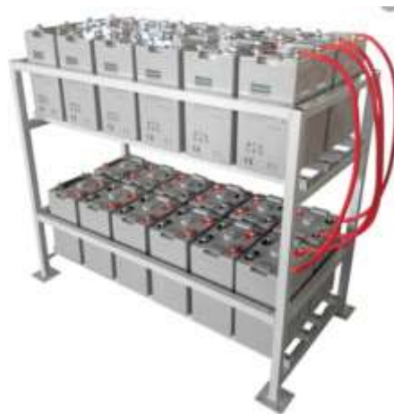
Fig.2.7 – The battery banks
