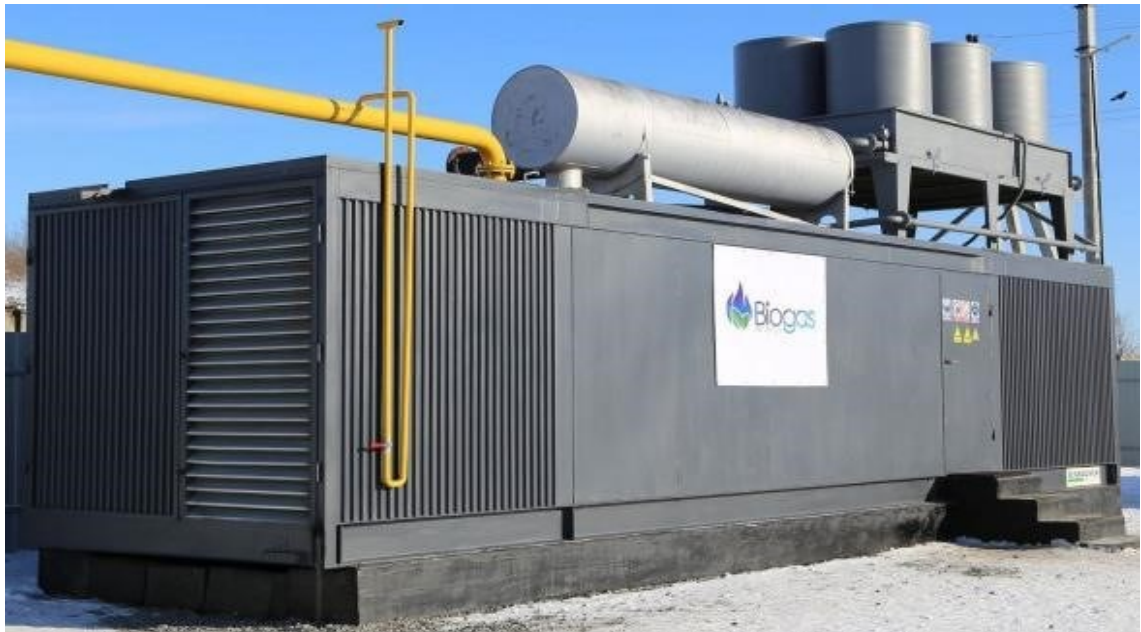
Fig. 3.1. Cogeneration plant in container design
